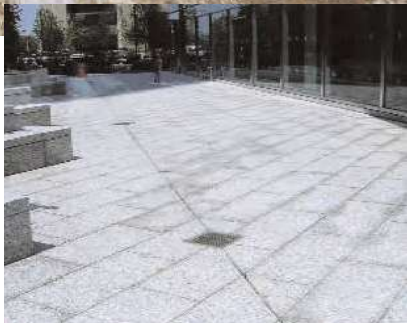
Moisture damage on exterior floor slabs.
